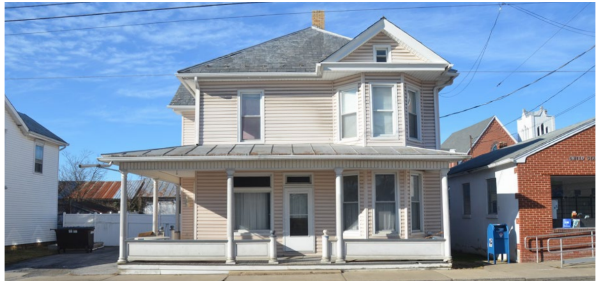
Some disadvantages of vinyl siding placed over wood siding include, but are not limited to: the concealment of any deterioration issues; corner trims and window surrounds that are not sized appropriately; and, an appearance that is “too perfect,” and therefore, doesn’t look authentic.
