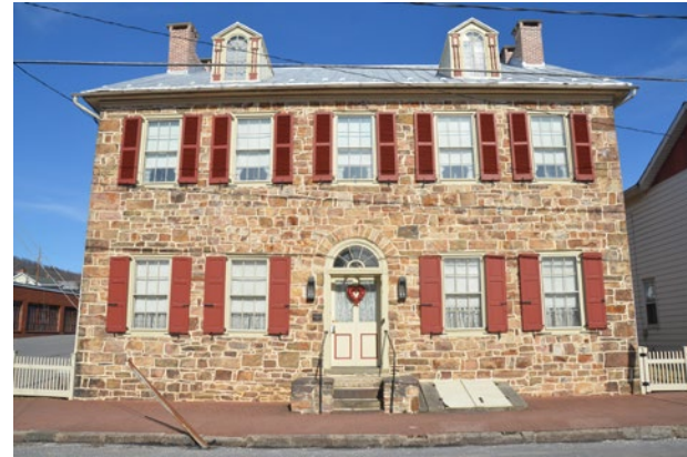
This residence in a nearby community does a great job of redirecting the gutters from the front façade to downspouts that go down the side façade.
