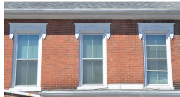
The careful design and placement of the storm windows maintains the character of the historic windows beneath.
