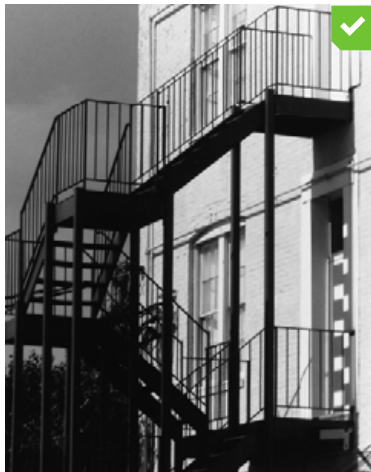
The placement of fire escapes at the rear of buildings usually is appropriate.
