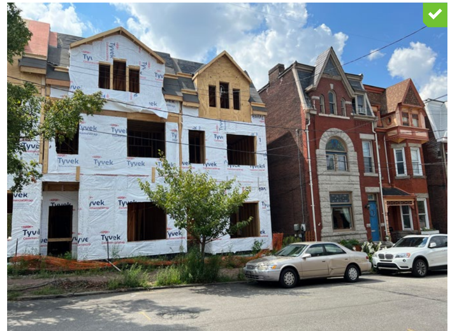
New residential construction in progress. Note how roof forms and overall massing relate to existing residential buildings.
