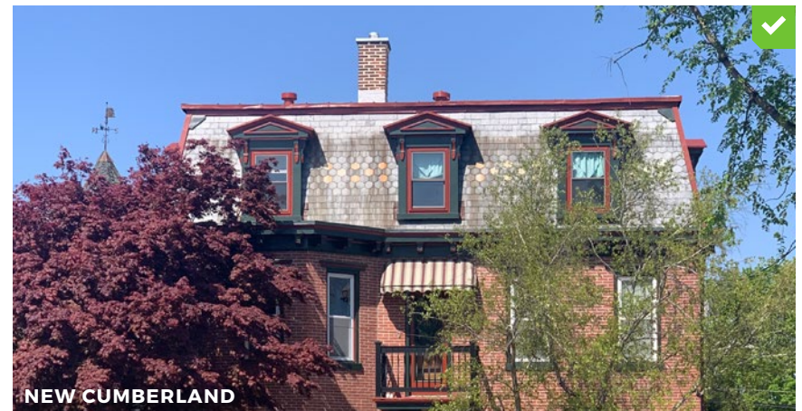
The preservation of original windows in their original shape and placement creates a harmonious appearance. The treatment could be improved, however, by painting the white frames a darker color to match the other window frames.
